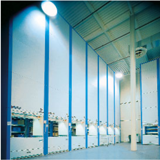
A typical installation from the Dynamic Storage and Retrieval Systems Division (KRM): a row of Kardex Shuttle units form a logistics solution for the centralized storage and retrieval of components and spare parts.
